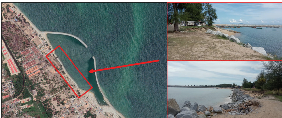
Figure 9: The jetty groyne of Tok Jembal facing shore erosion despite having revetment protection
