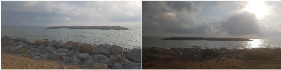
Figure 10: Revetment on the shore of Tok Jembal, with offshore breakwater on the middle of water
