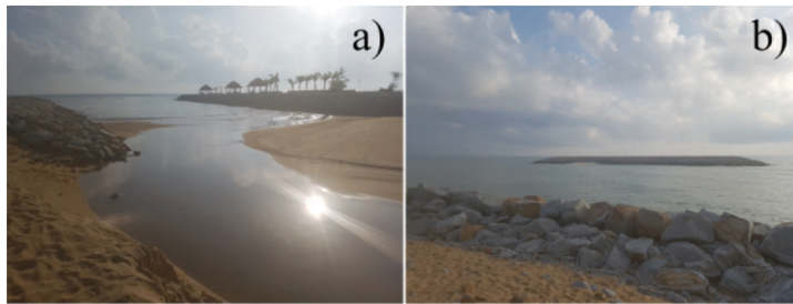
Figure 1: a) the groyne structure of Mengabang Telipot; b) The breakwater of Tok Jembal.
