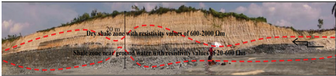
Figure 9: Soil slope located in Ayer Hitam Johor (Azhar et al. , 2016)
