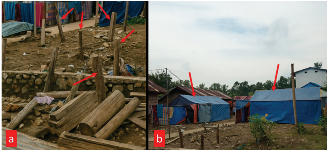
Figure 6: (a) Damaged house pillars after a flash flood, (b) Temporary evacuation tents in Wake Village Source: Authors (2024)
