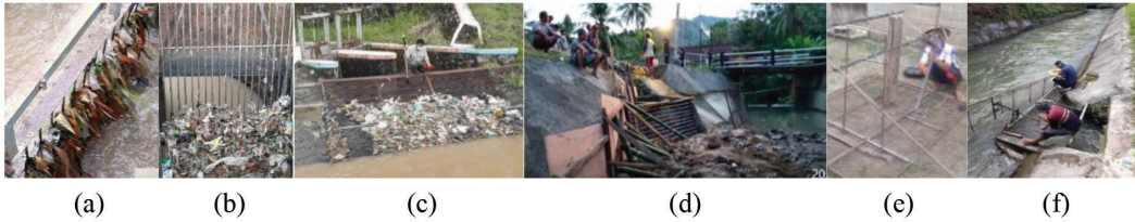
Figure 4: (a) Garbage in the Kalibawang irrigation canal caught on the trash rack of Kedungrong MHPP, (b) and (c) Diverting trash rack installed at the Kudungrong MHPP intake, (d) Widening of the intake mouth, (e) Construction of new trash racks and (f) Installing the trash rack at the trash rocker
